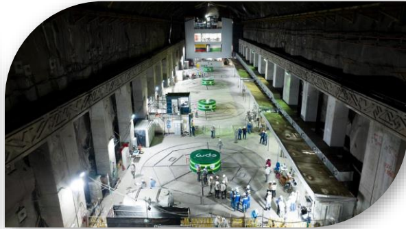
Powerhouse North Zone Units 1 to 4, 300 MW each
