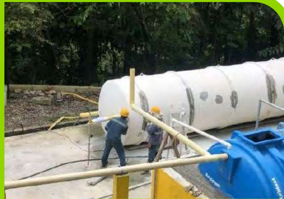
Expansion of the capacity of the domestic wastewater treatment system.
