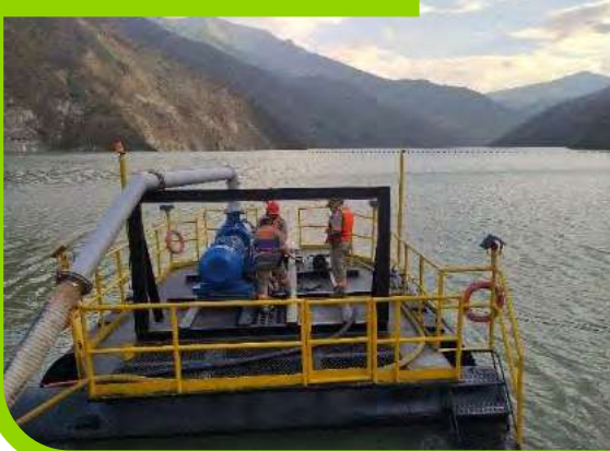
Adequacy of water pumping system for industrial use.
