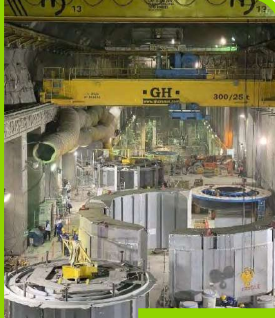
Rotors and stators of the generation units.
