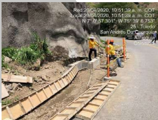
Construction of hydraulic work to allow the continuous flow of surface waters
