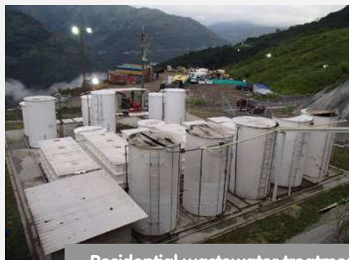
Residential wastewater treatment plant in Villa Luz camp
