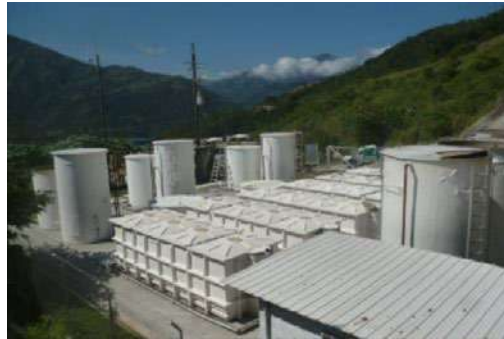
Residential wastewater treatment plant, Villa Luz camp
