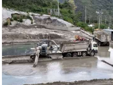
Operation of sedimentators and grease traps
