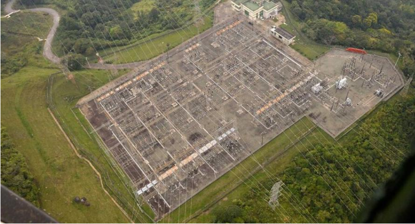
Guayabal 110 kV – 44 kV
